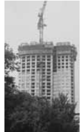
A view of The St. James at 34 floors on its way to 47 when complete.
