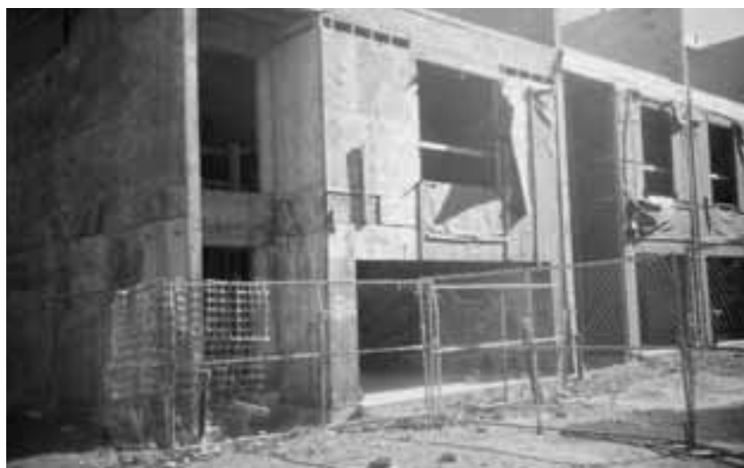
A New York developer will soon replace these derelict structures with new town homes architecturally compatible with existing historical buildings.
