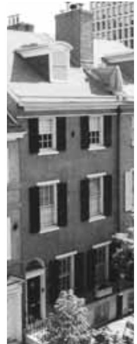
Under wraps: Tarps cover a roof repair gone wrong on Spruce Street.
