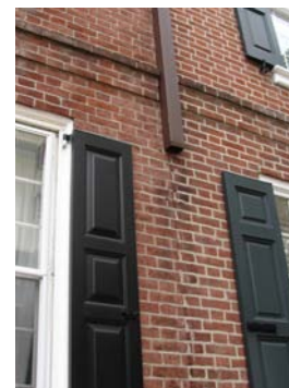
The site of one of many missing downspouts.
