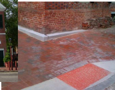
SHCA advocates for the preservation and restoration of its historic buildings and keeps tabs on current issues, halting the use of unsightly cheek walls and concrete ramp aprons in the ADA Project.
