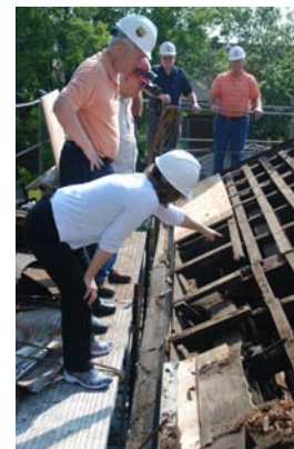
Parishioners and contractors examine the deteriorated trusses in the roof of St. Peter's Church.
