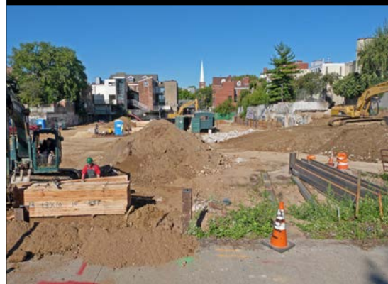
Work has finally begun at the Toll Brothers condo development, 410 South Front Street, projected to be finished by June 2015.
