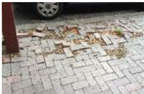
Dangerous sidewalks like these need repair.
