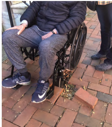
Wheelchair stuck in sidewalk.
