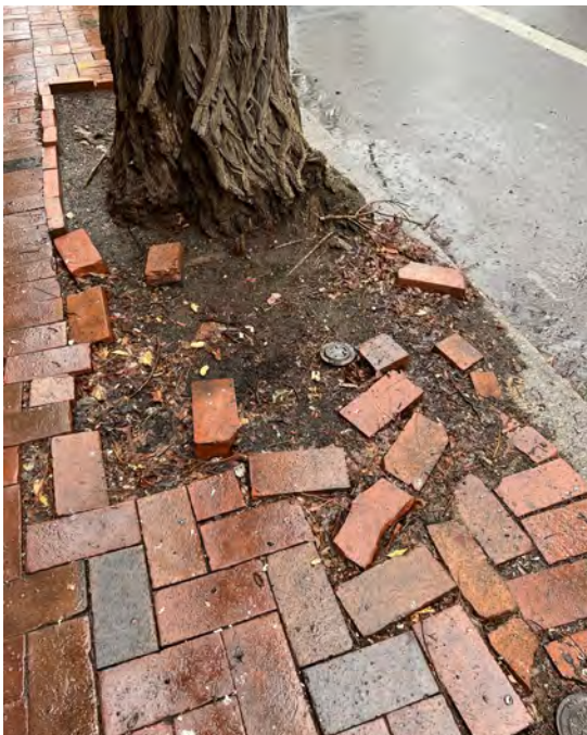
These loose bricks need to be secured or stored, not only for aesthetics but for safety concerns.
