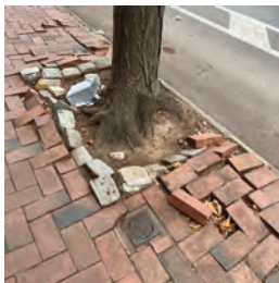
These loose bricks need to be secured or stored, not only for aesthetics but for safety concerns.
