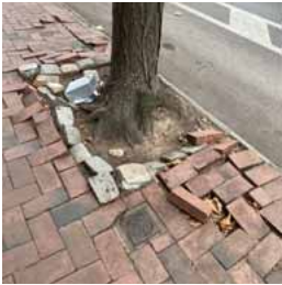
These loose bricks need to be secured or stored.
