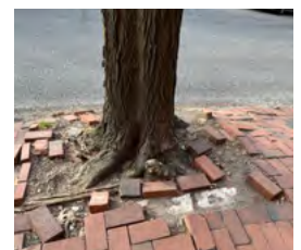
Loose bricks need to be secured or removed.
