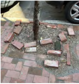
Remove and store loose bricks. Unsecured bricks like the ones pictured become tools of vandals.
