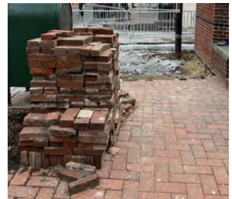
Dozens of bricks waiting to be replaced at 4th Street curb ramp upgrade.
