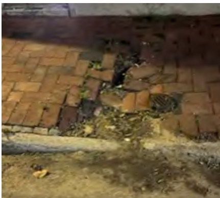
Loose bricks across the street from the Physick House.
