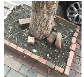
Loose bricks can be used for vandalism in the wrong hands. Remove or secure them in place.
