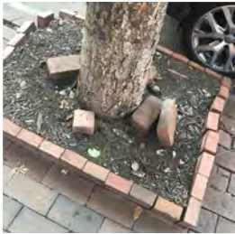
Loose bricks can be used for vandalism in the wrong hands. Remove or secure them in place.
