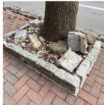
Belgian block is a tripping hazard.
