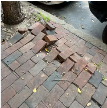
Tree roots can push up bricks.
