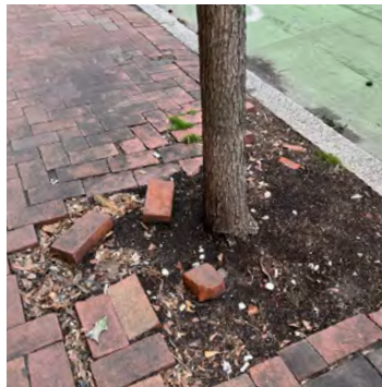
This tree pit is too small.
