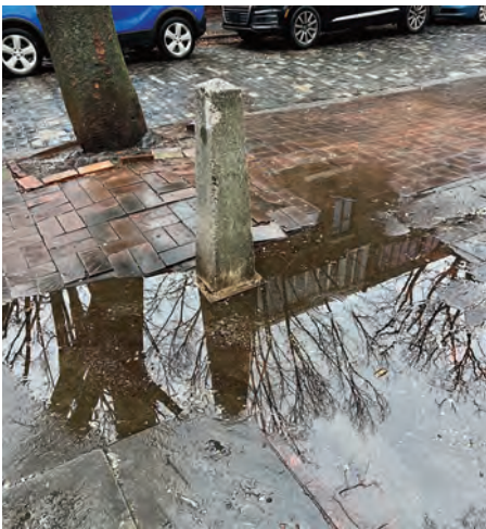
Pool caused by hump in sidewalk
