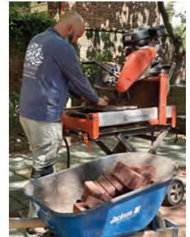
McFarland mason making ear-splitting custom cuts to bricks with a masonry saw.
