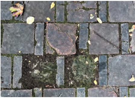
Damaged paving before restoration work began
