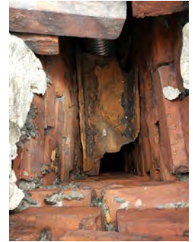
The broken clay liner inside this chimney needs to be replaced.
