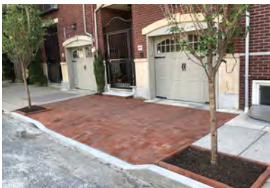
Fix your Bricks. Society Hill sidewalks should provide smooth, safe walking surfaces. The upheaval caused by tree roots can be corrected without removing or killing trees. Call McFarland to inquire about fixing your bricks.
